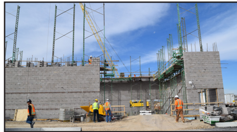
Quist Middle School construction started in June and will be finished in 2020. Pictured is the gym being built.
